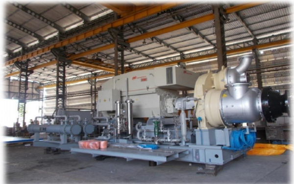
Air Compressor Package Client - Ingersoll Rand End User- Reliance Jamnagar
